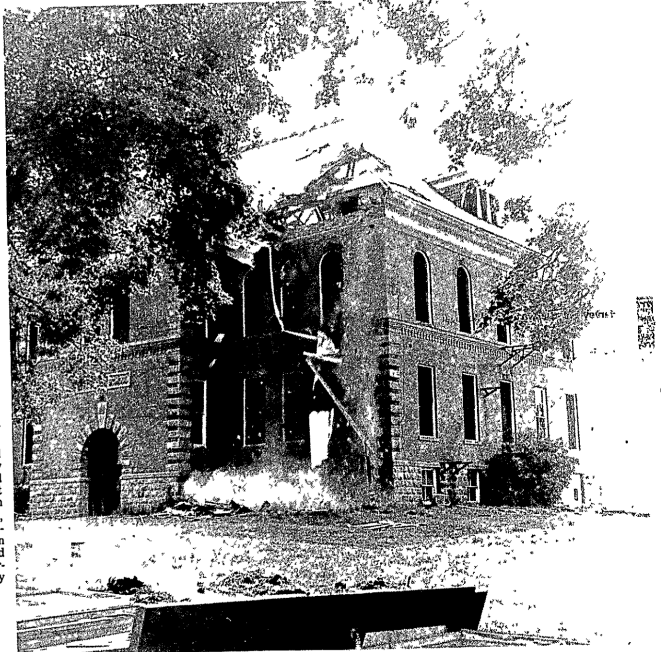
A bit of Elsie history was removed this week as the old Elsie High School was demolished. Although the school was termed deteriorating since 1950, workmen found removing the roof a difficult task.
