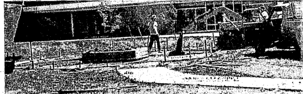
RUSSELL POPE (on tractor) and Tom Sutton work on the new student courtyard at St. Johns High School, sponsored by the St. Johns High School Student Council. Pope and employee Sutton donated material and labor for the courtyard. Walkways were donated by Martin Block who also provided a reduced rate for the courtyard concrete. Student Council president is Steve Kellen and Student Council advisor is Robert Koger. For Pope, the activity is familiar - he is the Ovid-Elsie High School Student Council advisor. Sutton is a junior high teacher in St. Johns.
