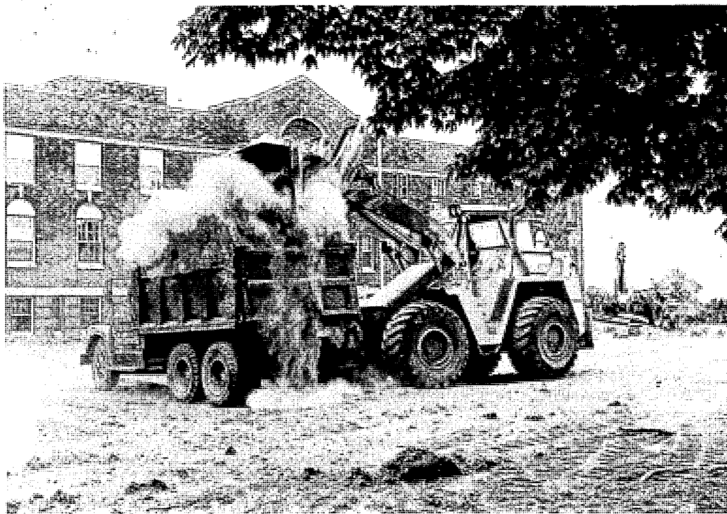
Work begins on new addition to hospital Contractors excavate dust from the front lawn of the Clinton Memorial Hospital in St. Johns Monday as work began on new $1 million additions.
