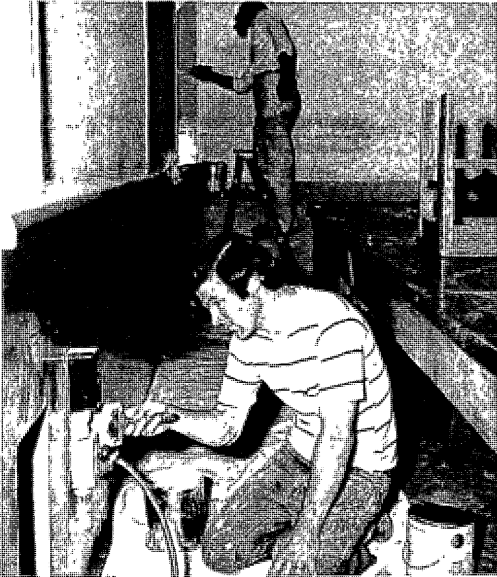
Terry Kentfield and father, Ray, in background, put the finishing touches on the walls of the art room at Rodney B. Wilson Junior High School.
