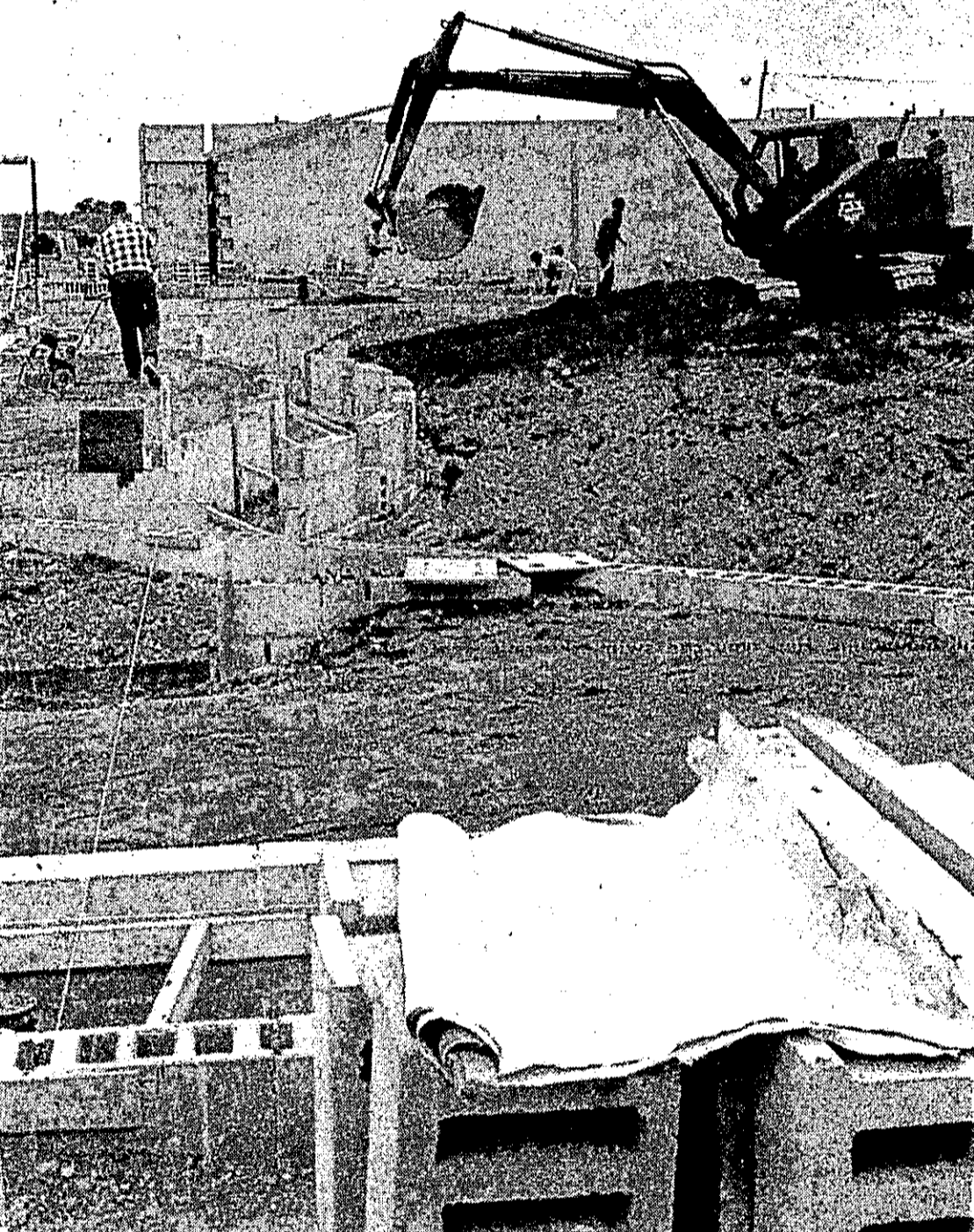
This portion of the new Ovid-Elsie High School will eventually be the auditorium-cafeteria. Last Wednesday contractors were working on the sub-floor facilities, moving toward the pouring of the concrete floor.
