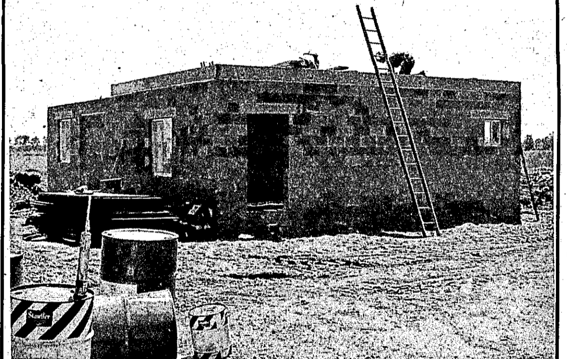
Kaufman Construction is building this new Milking Parlor for Frank Rivest on Watson Road.
