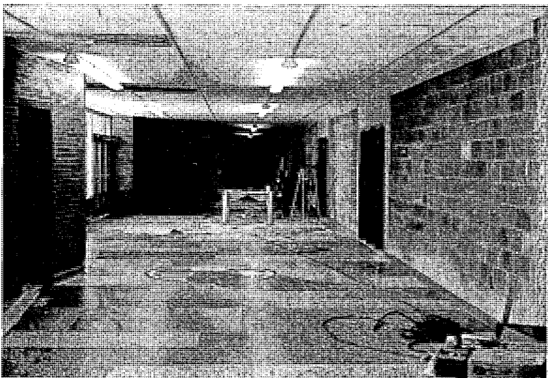
This is the lobby of the gymnasium at the new St. Johns High School, with the camera looking east. Notice the Redwing design in the terrazzo floor tile. The door at the left leads into a ticket booth. Back of the man kneeling in the background is a corridor leading into the cafeteria.
