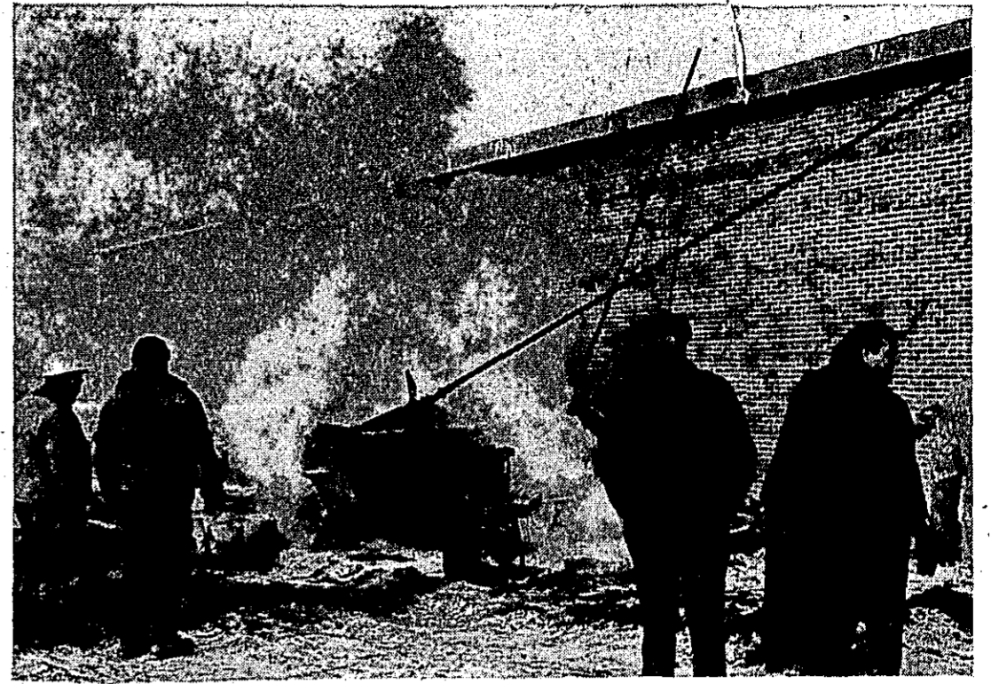
A blazing tar wagon, filled with tar for roofing work, was reduced to dense smoke last Thursday morning by St. Johns firemen, who answered the second of three fire calls to the new high school site this week. This fire seriously damaged the tar wagon; the other two involved no damage other than a tar mop which had apparently been set afire last Wednesday night.
