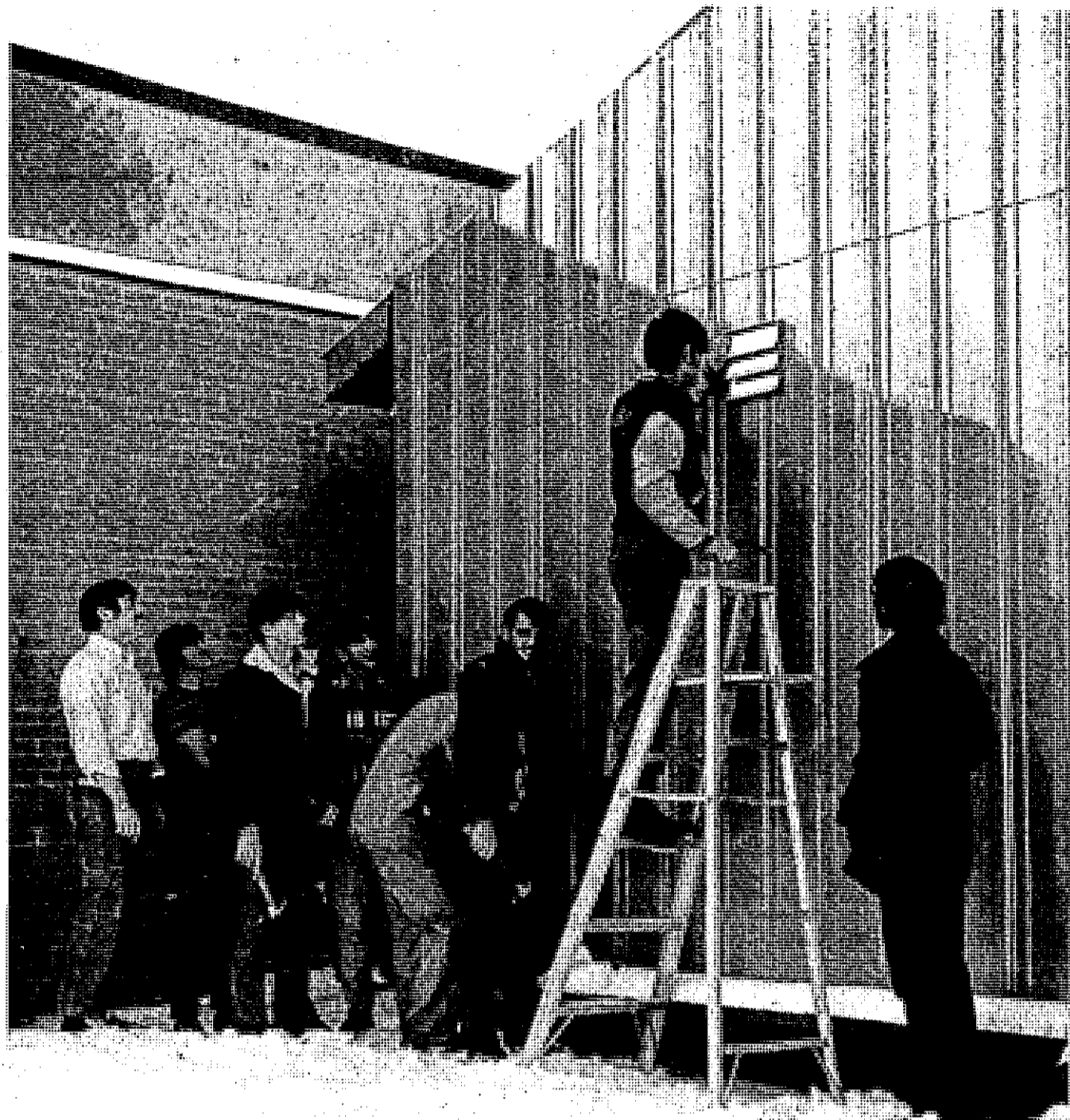
Members of the agriculture department course on animal science at Ovid-Elsie High School put the finishing touches to the outside of a special poultry building they constructed as part of their vocational educational program in agricultural mechanics. See page 15A.
