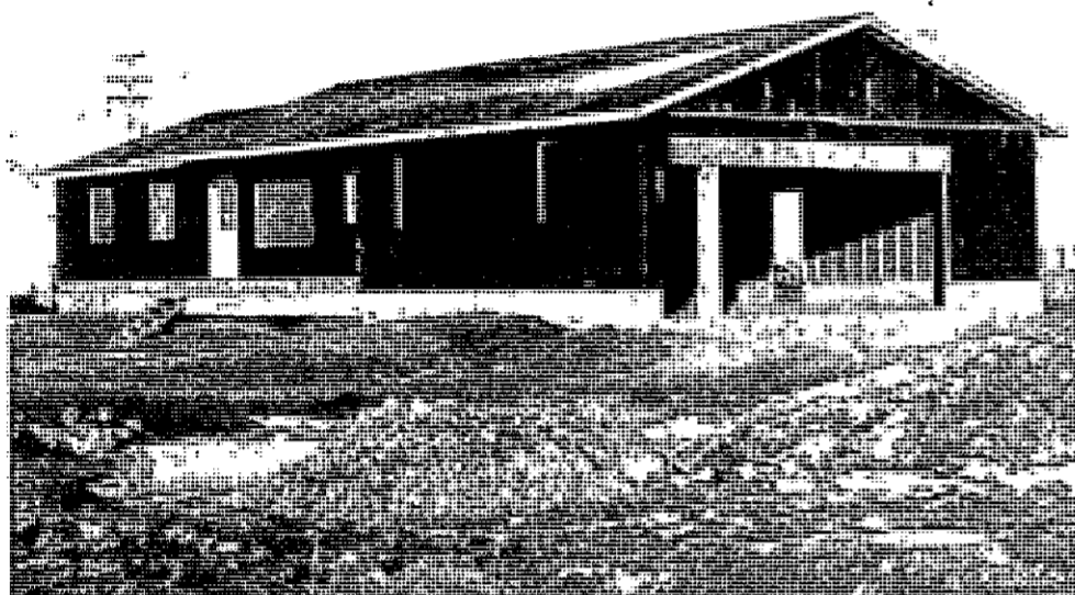
This is the house being built in Fowler by building trades as it looked in early stages of construction.
