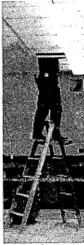
A "headless electrician" makes some adjustments to lighting fixtures in the new Ovid-Elsie High School.
