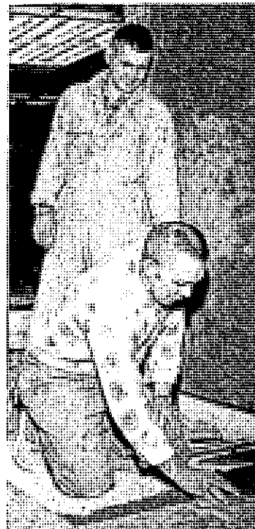
Entranceways to the library at the Ovid-Eastside High School will be tiled, and that's what these two workmen are doing.
