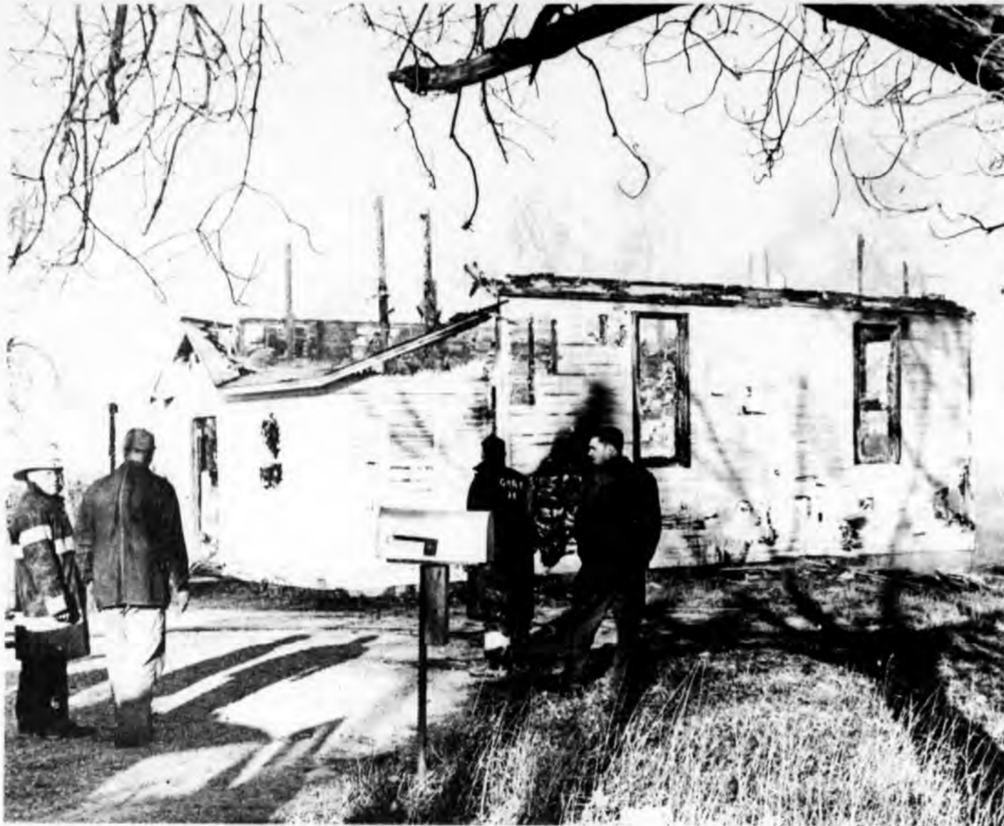
St. Johns firemen and neighbors stand by before pushing down the walls of the burned out Marshall School just off US-27 in Greenbush Township. The school burned Saturday morning with the loss estimated by firemen at $5,000. Cause of the fire was believed to be defective wiring.
