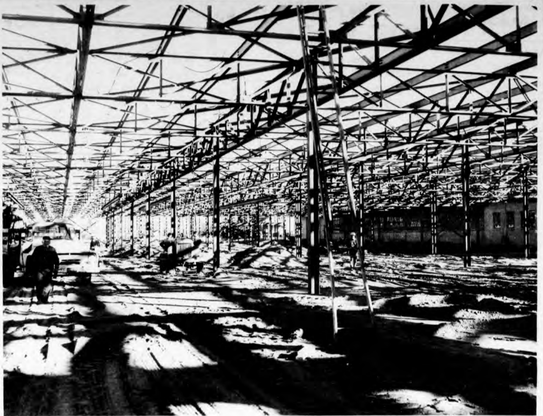
Steel Work Forms Variety of Patterns in the New Addition to Federal-Mogul Plant in St. Johns
