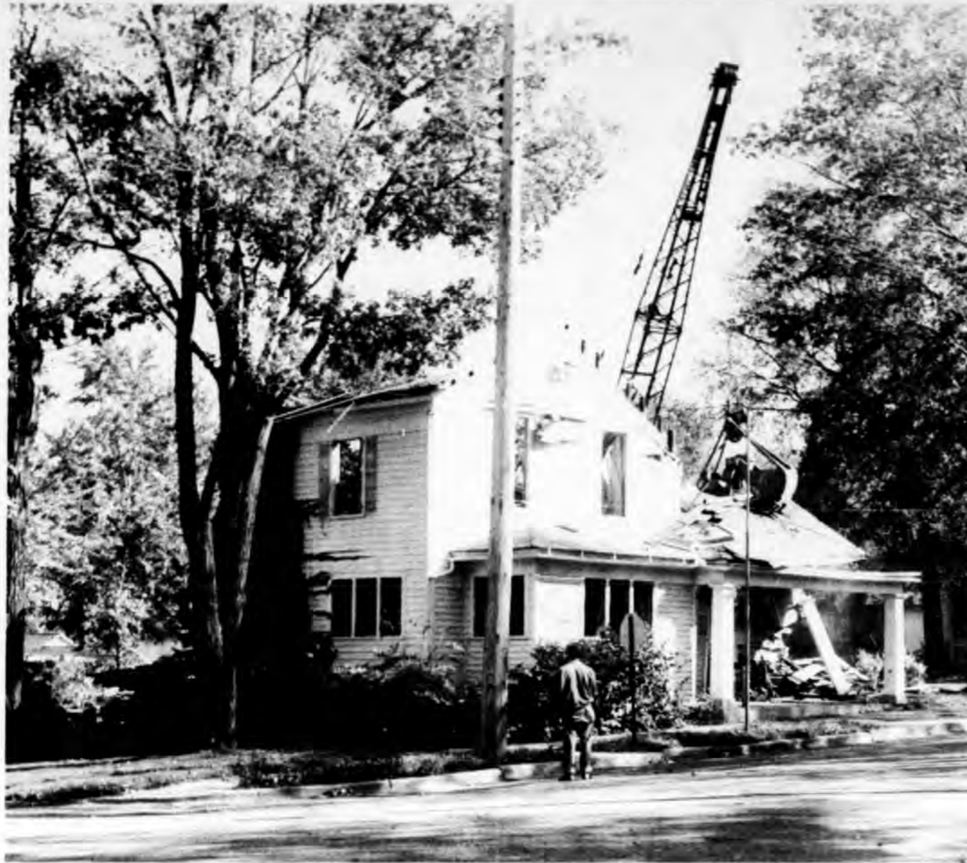
The big bucket of a crane takes a big bite out of the former funeral home at the northeast corner of Spring and Walker streets. The building was razed Saturday morning by the Central Wrecking Co. of Lansing, a firm owned in part by Jack Smit of St. Johns. A new building for the new Central National Bank will be constructed on the site. The old home was torn down in 4 1/2 hours.
