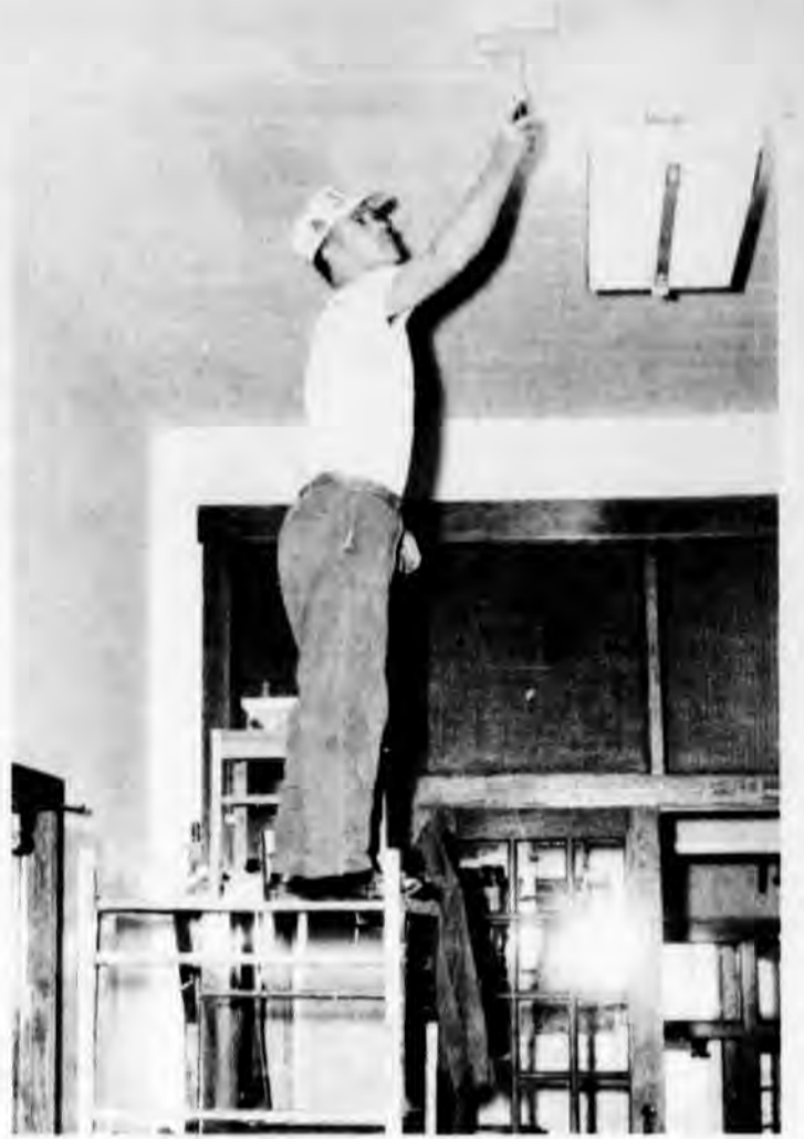
Work on the interior of St. Johns High School includes painting of ceiling tile with fire-resistant paint. Robert Gilbert is shown here painting in the school's front entrance hall.
