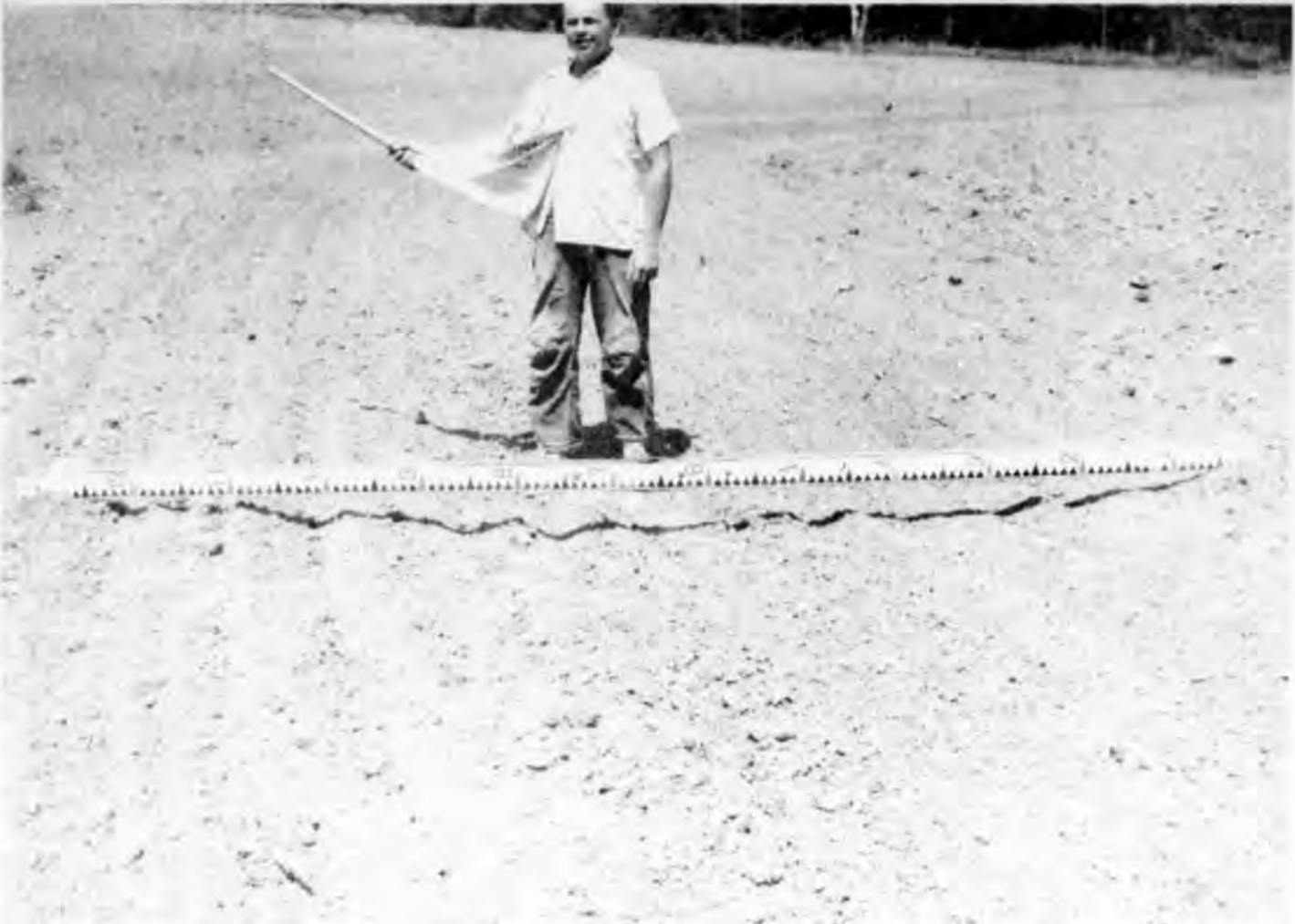
Lawrence, 18-year-old son of Umbra Pierce, stands in a newly constructed waterway on their farm in southwestern Essex Township. The waterway is being checked for proper design before seeding and mulching. The Pierces are building 99,000 square feet of waterway this month.
