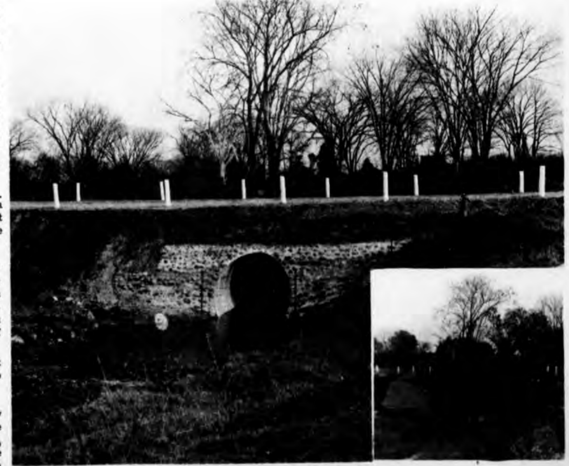
On Forest Hill Road South of Colony Road View of old bridge (inset lower right)
