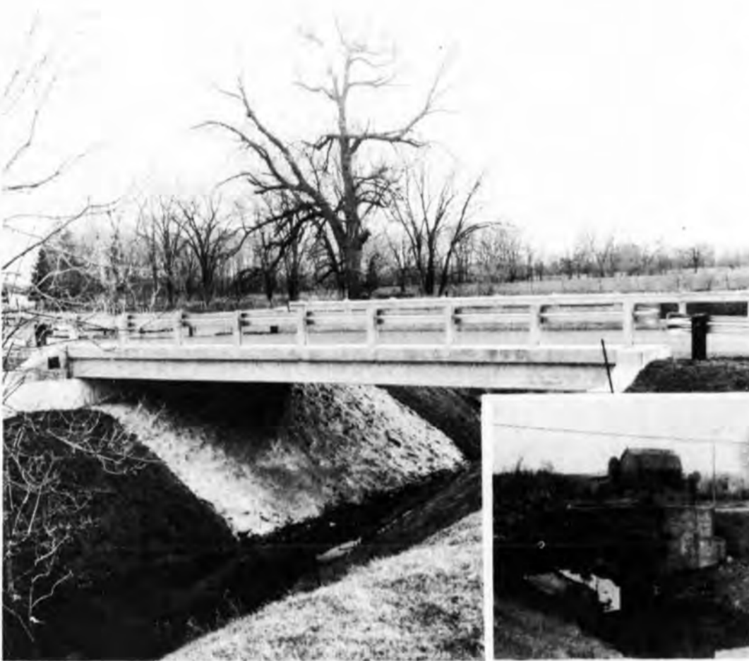
On Clark Road Crossing Remy Chandler Drain View of old bridge (inset lower right)
