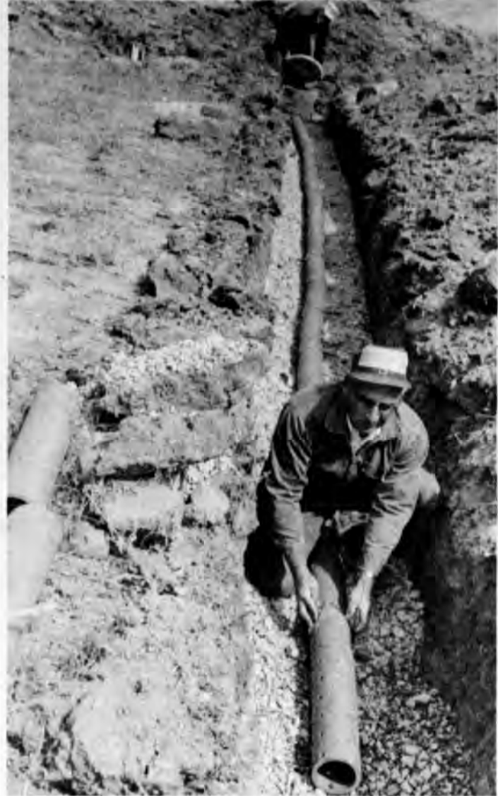
Wendell Waggoner of Randolph's Re-di-Mix Concrete works over tile being laid in the field of Loren VanOstran (shown in background).
