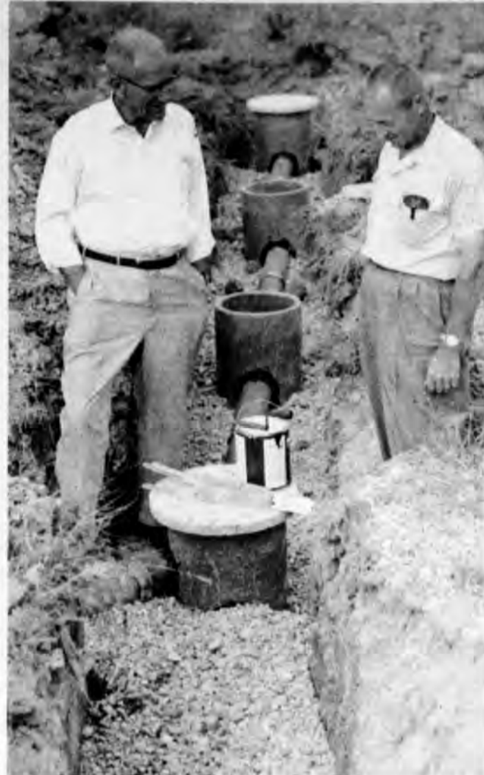
George Amundson (left) and Gerald Shepard look over the work being done in VanOstran's field. Amundson made the layout for the septic field.
