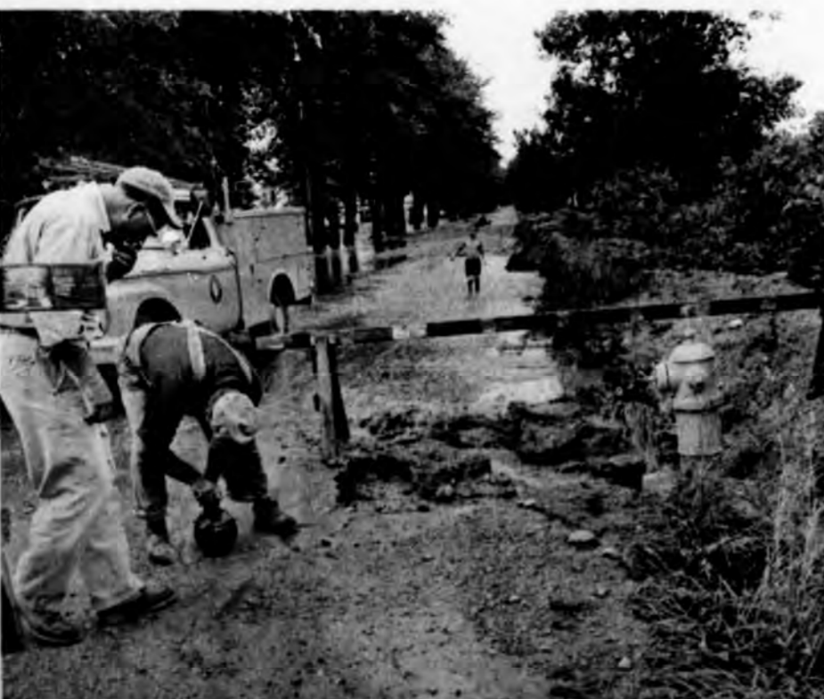
PART OF SOUTH Lansing street in the 900 block washed down into a field to the east. Warning devices were put out.
