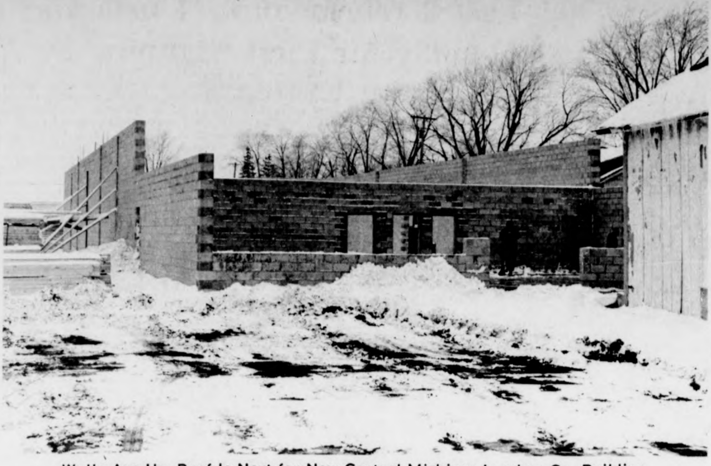
Walls Are Up, Roof Is Next for New Central Michigan Lumber Co. Building
