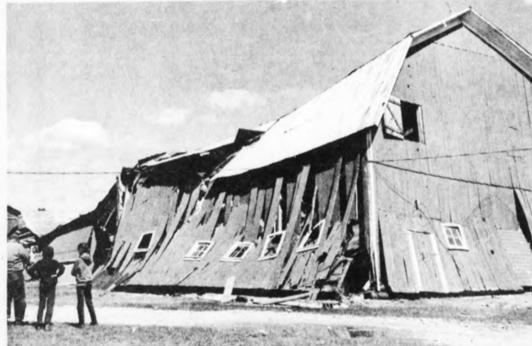
A very strong gust of wind or a brief and small tornado demolished the barn belonging to Edwin (Joe) Brown on North DeWitt Road late one August Friday evening.
