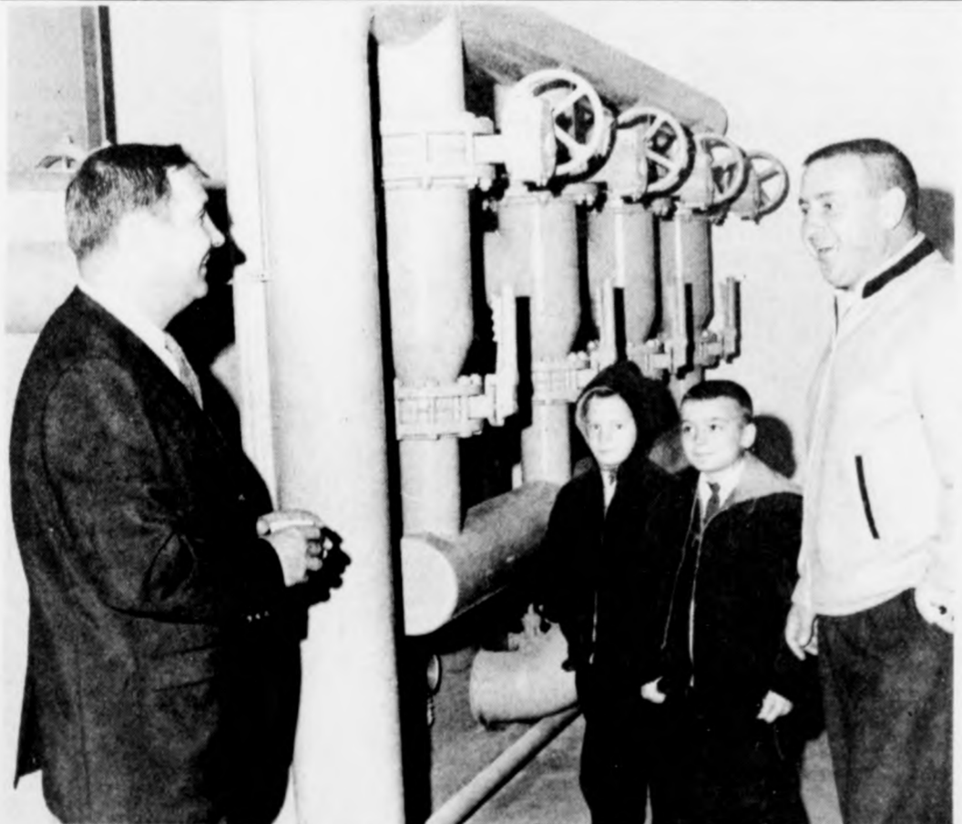
Ovid Councilman Joe Michutka explains the operation of Ovid's new water treatment equipment to Paul Binger of Ovid and his sons Randy, 8, and Paul, 9. The Bingers inspected the plant and public works building Sunday during an open house.
