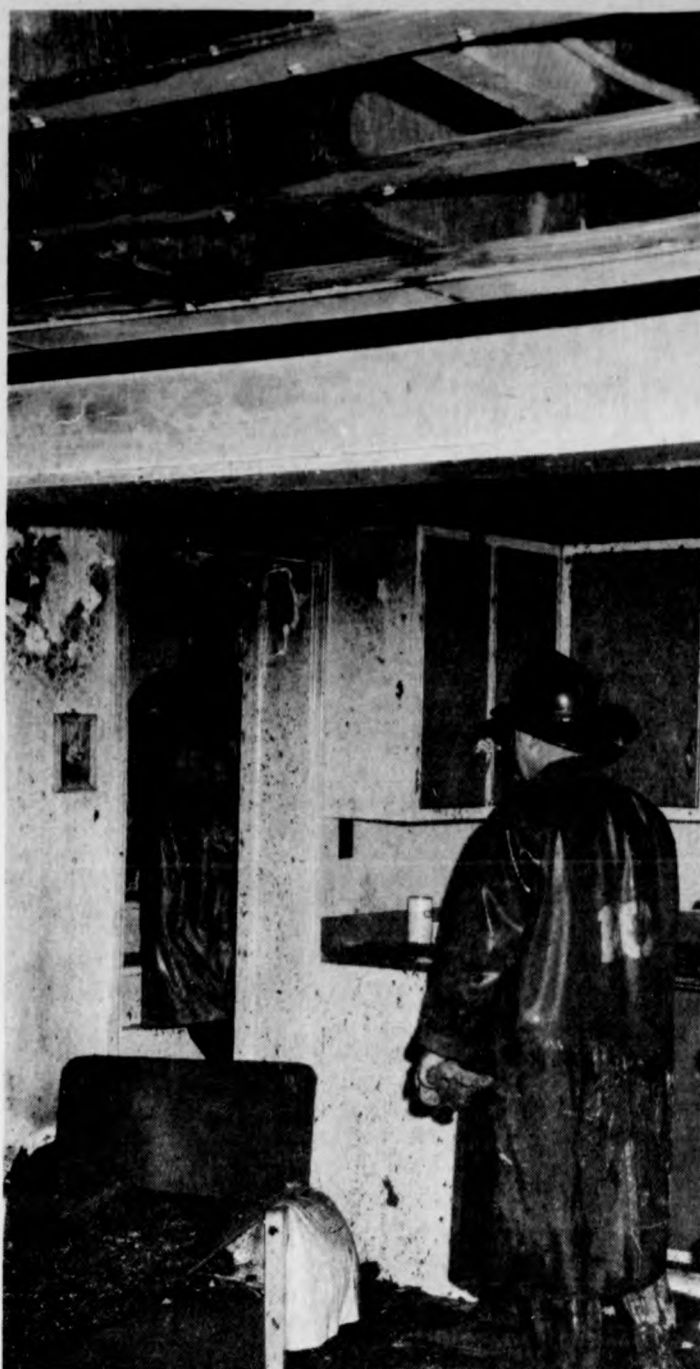
Fire Guts DeWitt Area Home
