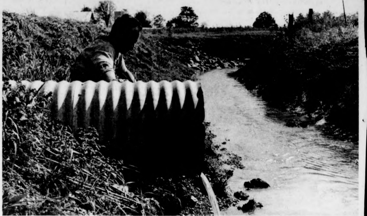
Greenbush Township farmer John Jones checks his 21-inch corrugated metal pipe, which is connected to a concrete drop box erosion control structure. Jones has a good stand of ditch bank seeding only six weeks old on the bank in the background. Stone rip-rapping along the left bank also protects the open ditch.
