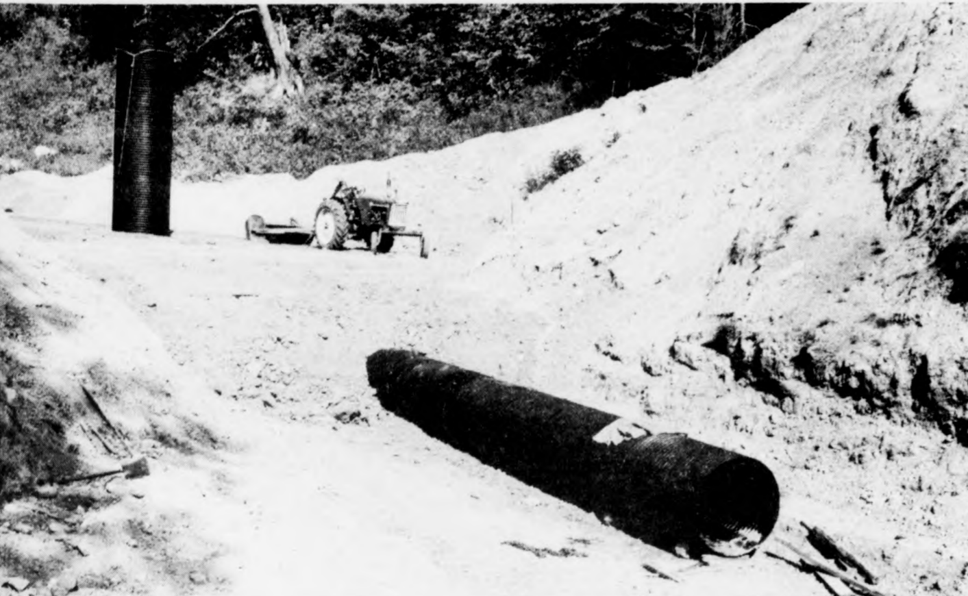
This picture of the Keith Wright farm pond dam site shows a 42-inch outlet pipe with soil mechanically tamped. A 60-inch-diameter riser pipe will result in water 20 feet deep when the dam is completed.
