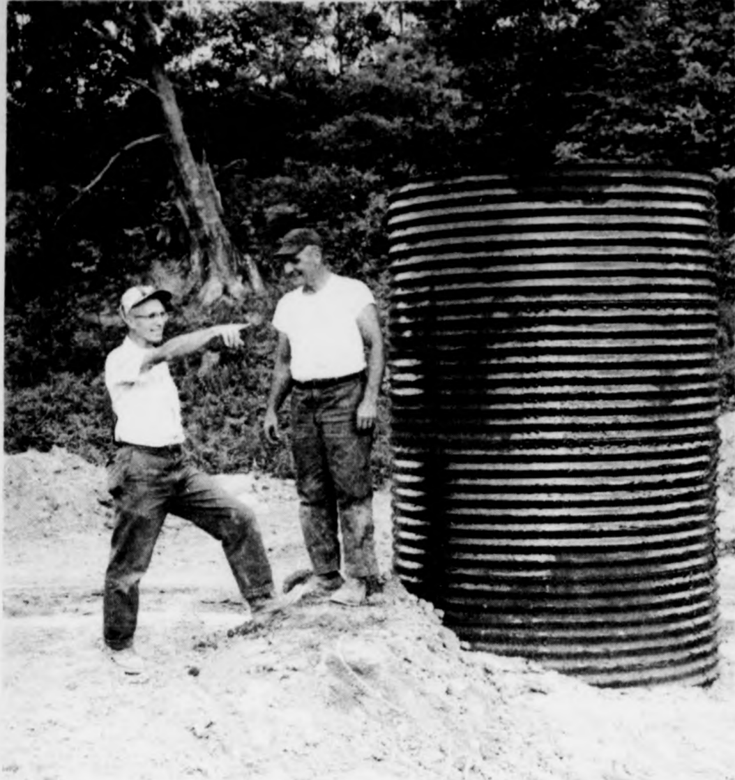
Keith Wright (right), owner, and Orville Beachler, soil conservation technician, discuss compacting the fill around a 60-inch riser pipe during the construction of a dam for Wright's new farm pond.
