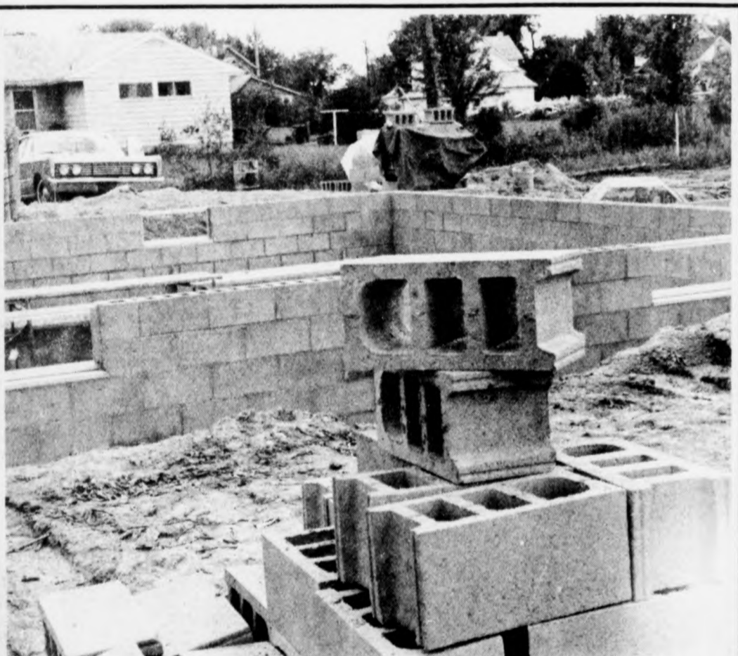
Another new home basement being constructed with KARBER'S CONCRETE BLOCKS. This one is being built by Kingsbury and VanEtten, contractors, is located in the 800 block of East Walker Street.
