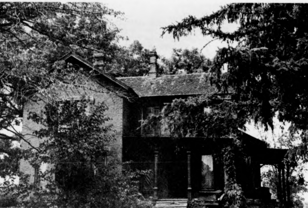
This is the Fred Barber house on Jason Road near Lake Victoria, repeated target of vandals during the last six months.
