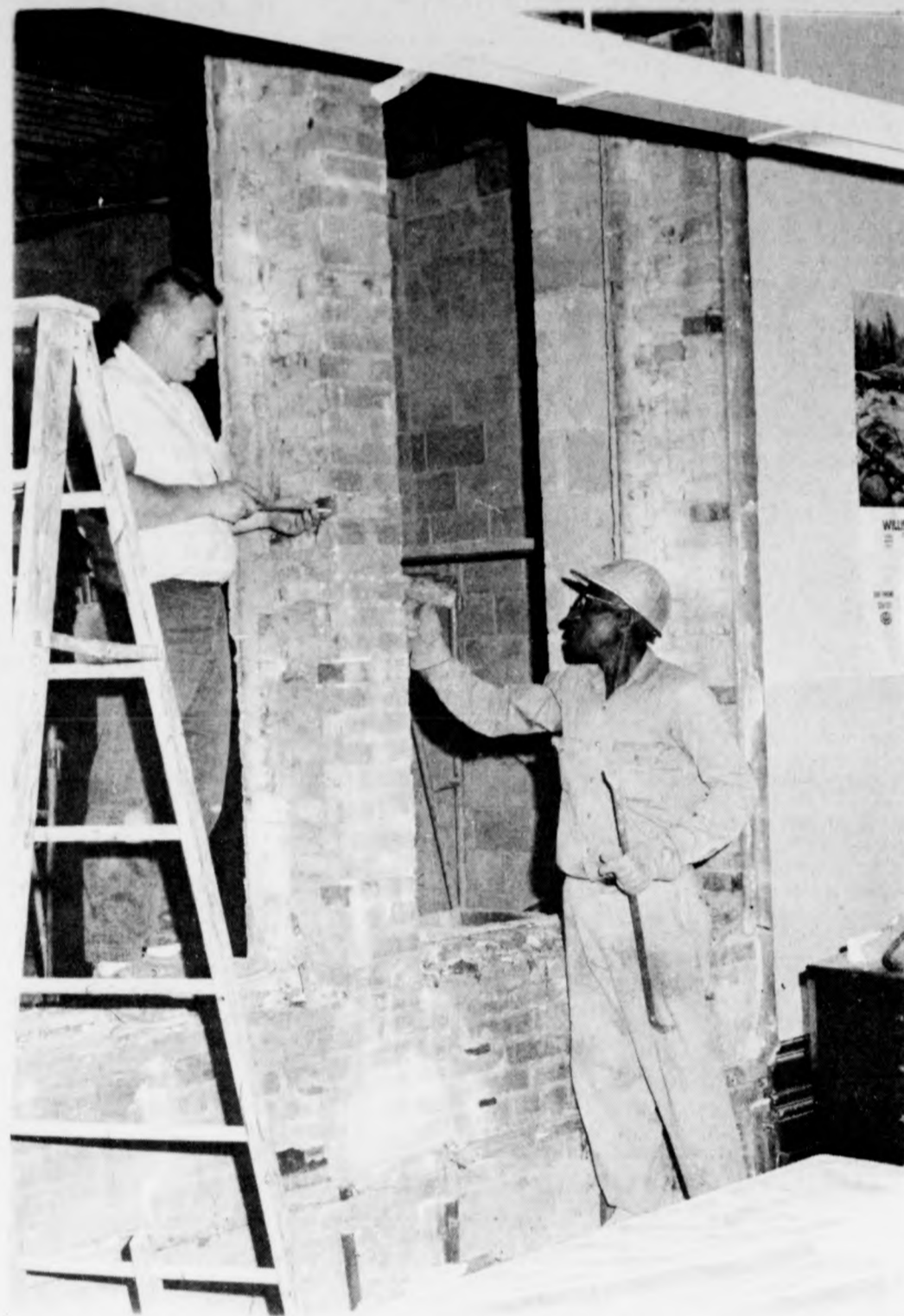
Lowell Martin (left) of the Pittsburg Plate Glass Co., and Horace Cameron of Granger Brothers Construction Co., work at removing a window casing on the former west side of the county clerk's office preparatory to making an archway entrance into a new section of the office. Clerk Paul Wakefield and his staff have been holding fort in the probate courtroom while the connections are made between his office and the new courthouse wing.
