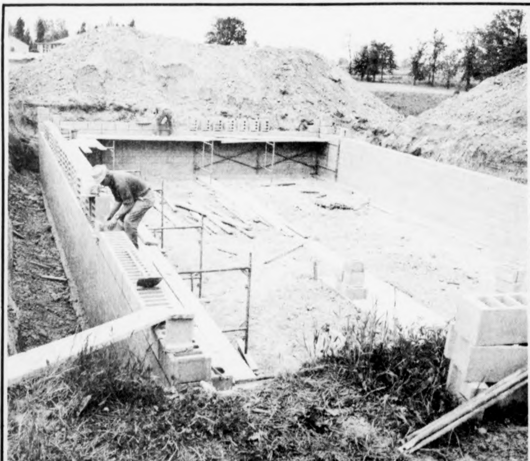
Richard Cornwell, St. Johns Building Contractor, is pictured at a home construction site on Wildcat Road. Karber's Concrete Blocks were used for construction of the basement.
