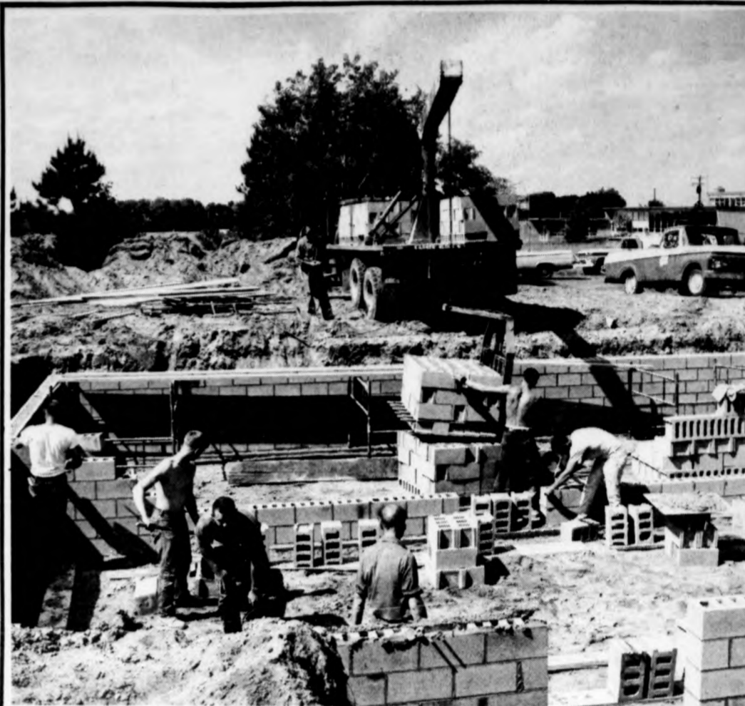
Kaufman Construction Co. takes full advantage of Karber's Side-O-Matic Delivery. Pictured above is a load of blocks being lowered into the basement of a new home being constructed in Elsie by the Kaufman Construction Co.
