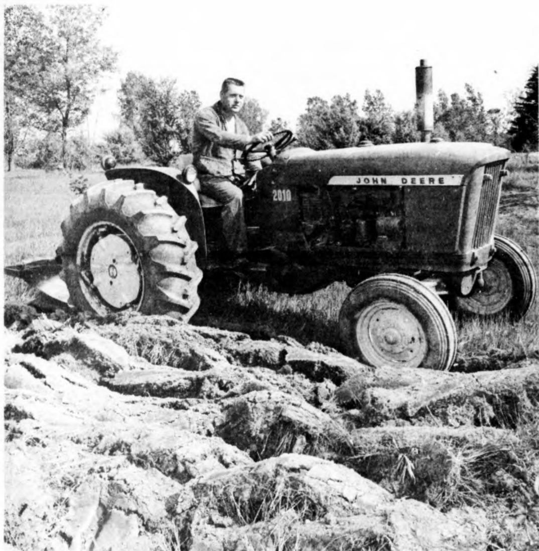
In some places plowing and reworking of the terrain were necessary. Jaycee President Dan Martin mans a tractor on one of many Jaycee work parties at the site.
