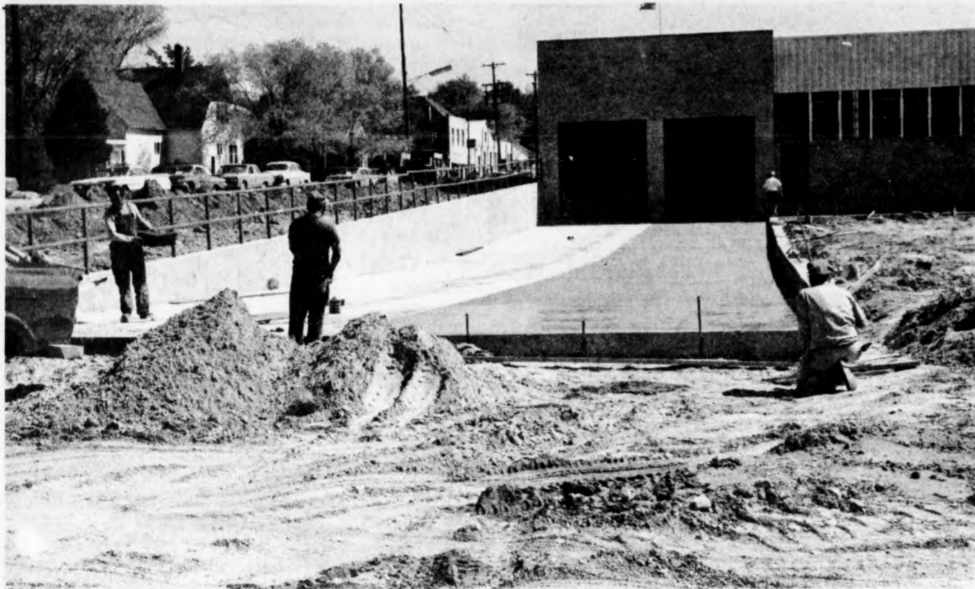
Workmen tidy up after a fresh pouring of concrete on the ramp for one of Federal-Mogul Corp.'s new loading docks in their new addition. Curbing leading into the giant parking lot is also in.
