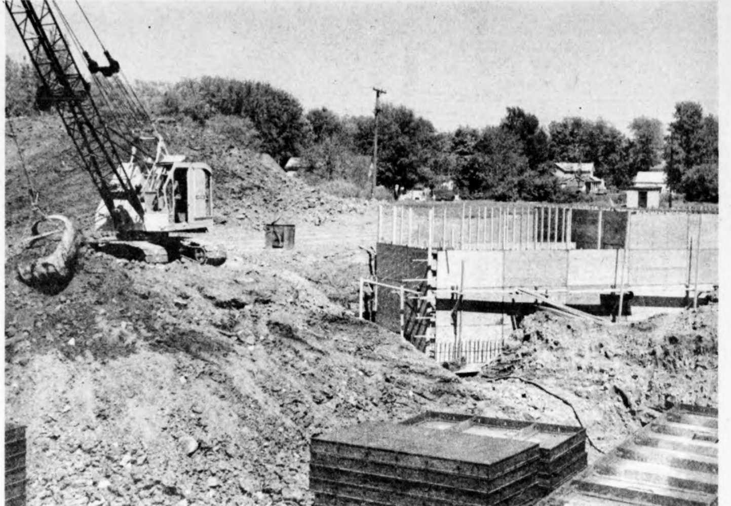
The big pile of dirt in the background came from the big hole in the foreground as work progresses on the new St. Johns Water Treatment Plant off Lansing Street between Lewis and Gibbs Streets. Forms for the plant building itself rise at the right center of the picture.
