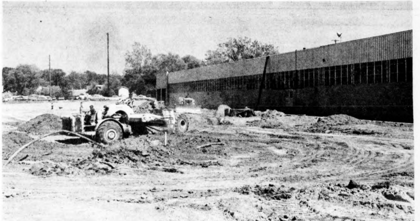
A big earthmover scrapes up dirt from the future Federal-Mogul parking lot next to the new addition. The lot has been leveled off in preparation for use of the lot.
