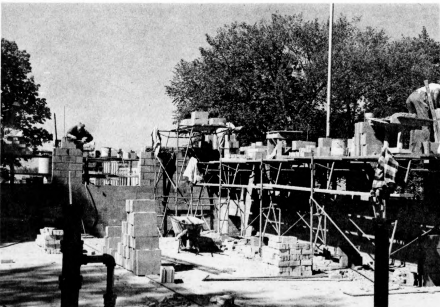
Bricklayers, bricks and scaffolding are the common sights at the Clinton County Courthouse these days as the walls rise higher.
