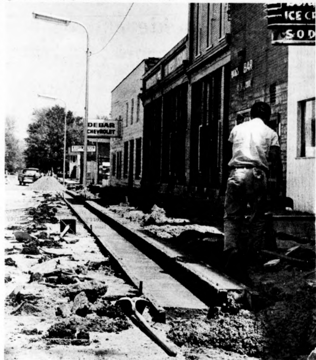
A workman tends to his cement work on new curbing in the Elsie business district Friday. Other visible signs of Elsie's springtime improvements are a new sidewalk on the south side of the street and new boulevard-type street lights in the business district. The new lights are already in use.
