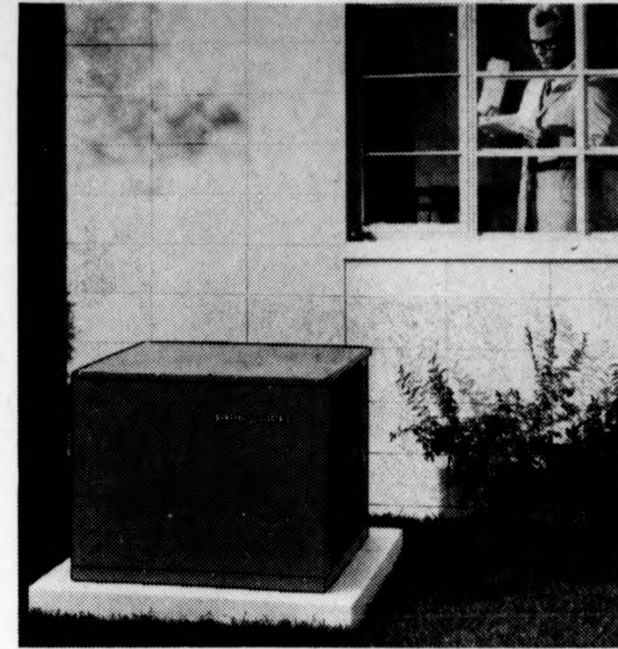
ONE THERMOSTAT CONTROLS BOTH air conditioning and heating, with a heat pump at work to provide year-round comfort. System shown here is powered by an outdoor unit that is unobtrusive and can be neatly located near the home. Weathertron system by General Electric.
