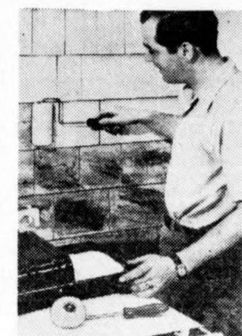
SLICK-UP jobs on exterior sidings can have that professional look with a once-over wide roller, plus a "donut" roller for under edges of lap. Roller covers of Dynel modacrylic fiber.
