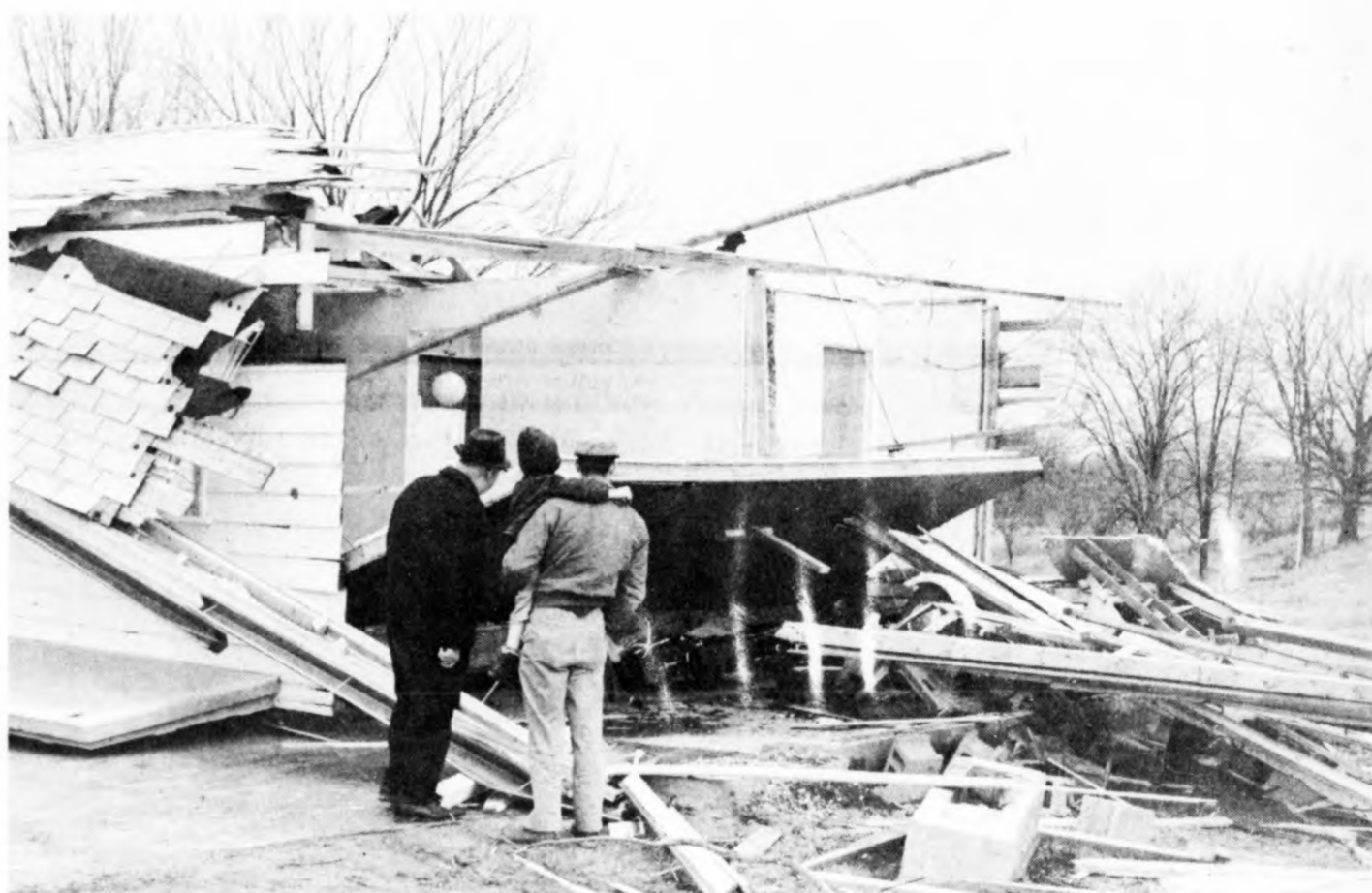
Neighbors and friends look at the wreckage of the John Bates home at the far end of Theresa Street, the street hit hardest by Sunday evening's tornado. The garage and part of the east side of the house were ripped and torn away from the rest of the structure. No one was home here when the storm hit.
