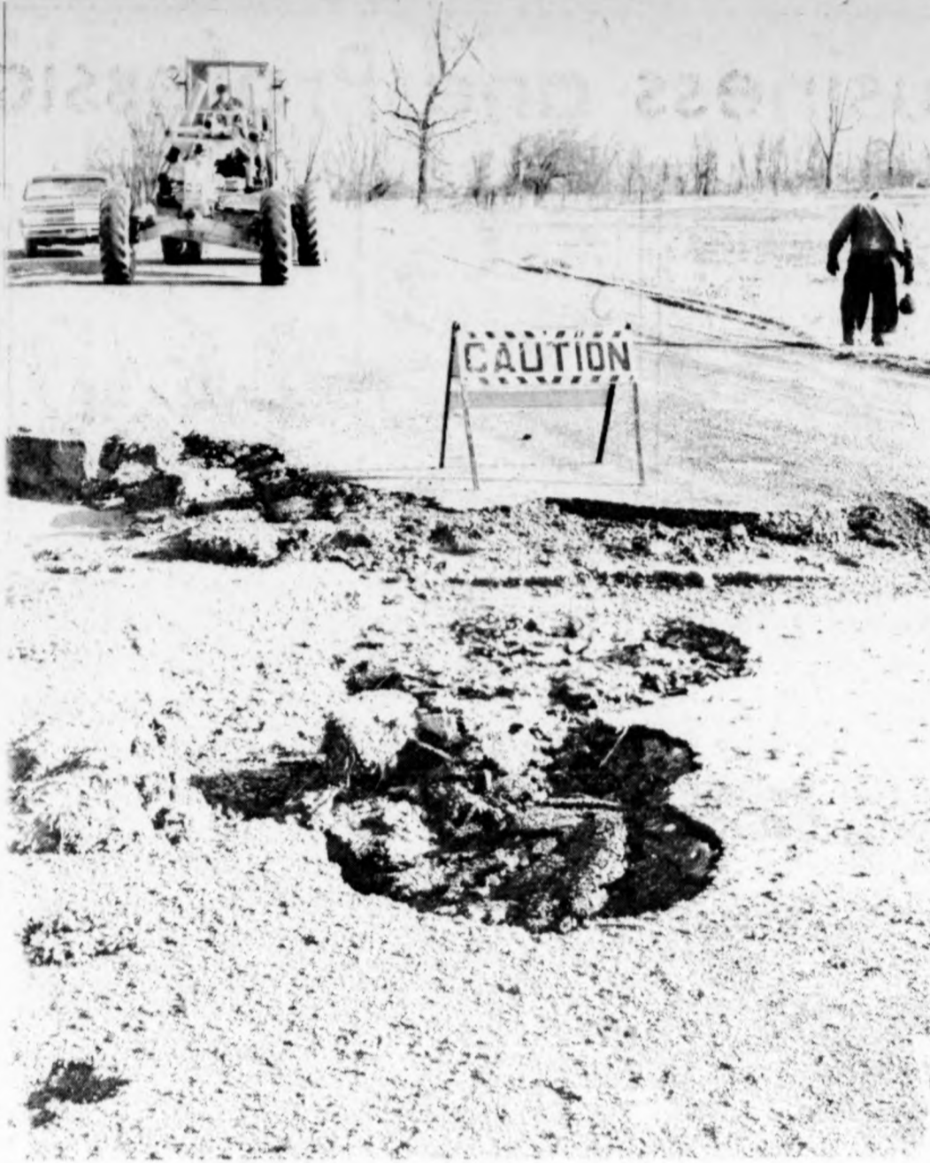
Washed Out Result of Massive Thaw
