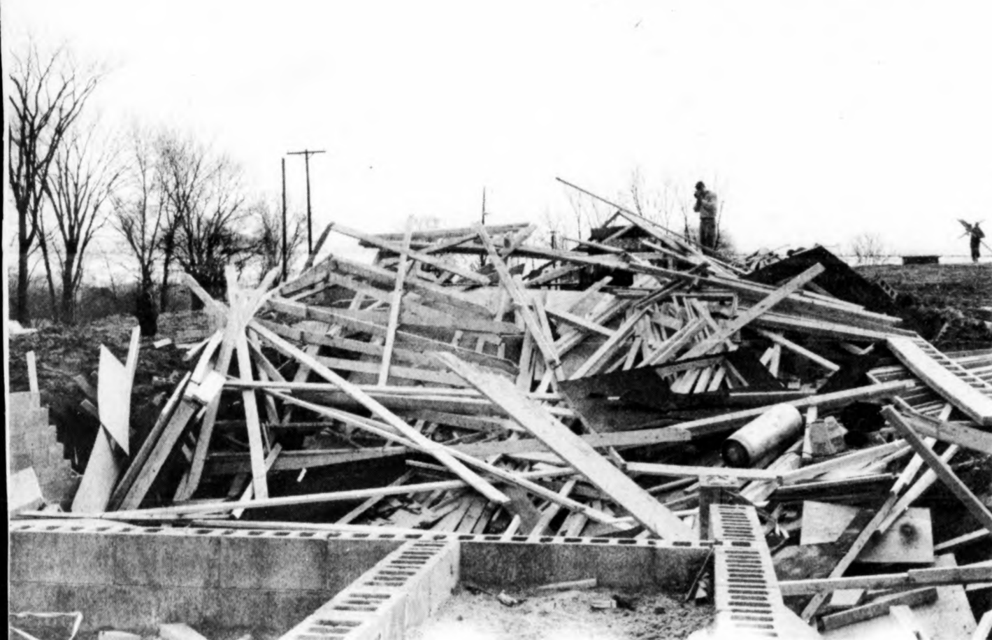
This was a home under construction on Clark Road south of DeWitt before it fell in the path of Sunday night's tornado. Contractors said the house was ready for the dry-wall to be installed. The twister reduced it to kindling.
