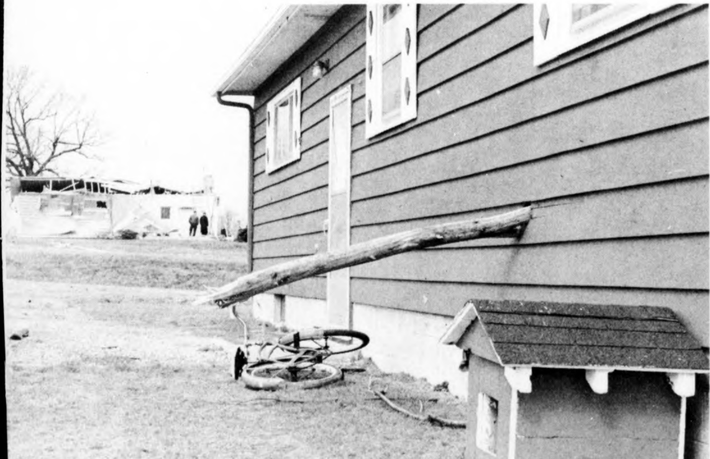
A six-foot limb off a tree in a nearby woods pierced the siding of the Louis Sipka home on Theresa Street, causing the only damage to the house in Sunday's tornado. Another foot or so of the limb reached into the Sipka's bedroom. The house in the background belongs to Henry Dreps; it was one of five destroyed.
