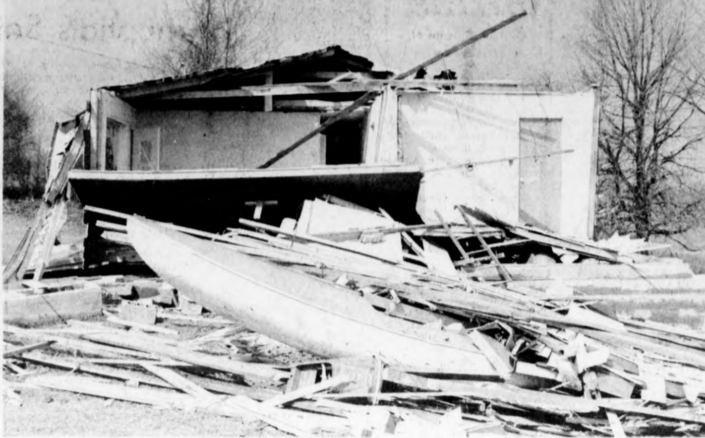
Boat Left in Garage Damaged, Too, As Twister Wrecks Home
