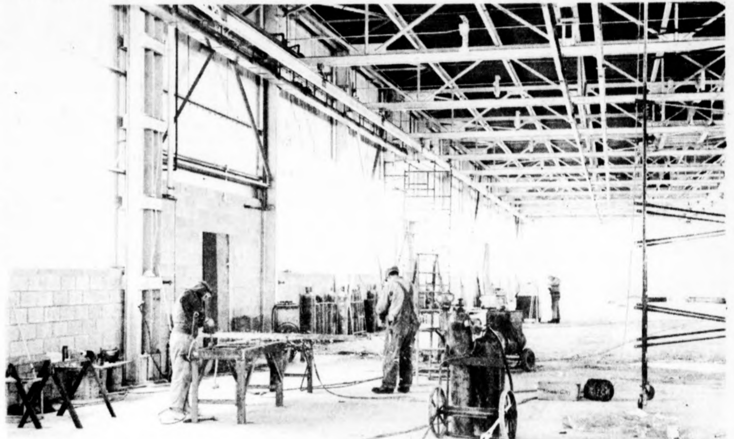
Sparks fly as worker at left and others put the final touches on the L-shaped building that is the new home of the Ashley Corp. at Ashley. With completion of the building, fabricating equipment will be moved in and the company will begin manufacturing of railroad car equipment. The building is 300 feet long and 120 feet wide.
