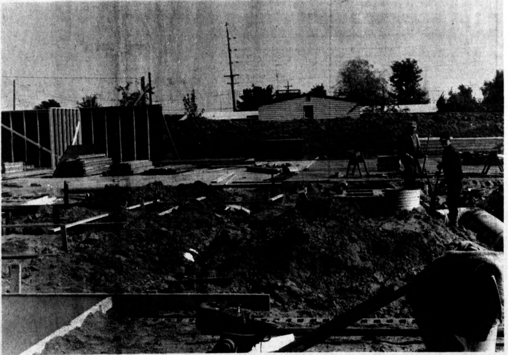
Work is moving right along for the new county office building which is being constructed behind the county annex on Oakland St. Various activities are being done from bulldozing, to pouring cement, to putting up walls as seen in the foreground. The building is expected to be completed sometime after the first of the year.
