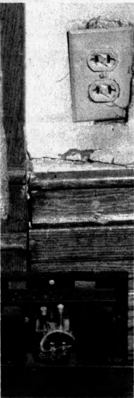
Cracked outlet and exposed telephone equipment reflect conditions in Health Dept.
