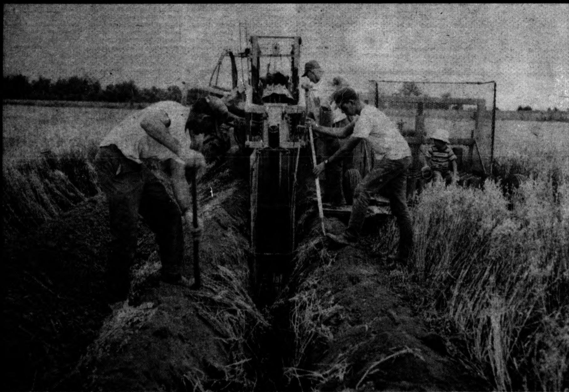
Stanley Thelen and his son fill in top soil over his four-inch lateral being installed by Platte Brothers. This 20-acre field was tiled every five rods. Installing tile drainage every four yards costs a minimum of $250-$300 per acre, but Clinton County farmers feel it's worth it. Over 1 million feet of tile was installed on Clinton County farms in 1976. It is reported that yields from tiled fields are 20 to 25 percent higher and can pay for a tiling project in three to five years. You can learn more about tiling and other soil conservation practices in this 1977 edition of the Clinton County Soil Conservation special section.
