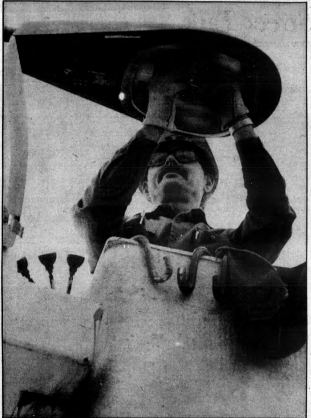
If you thought it was a pain to change the bulb in your lamp, imagine what John Kabustka of Consumers Power has to go through when he changes the street lights in St. Johns. Kabustka was in his cherry-picker Friday afternoon, helping keep the city bright. (Photo by Bob Stern)
