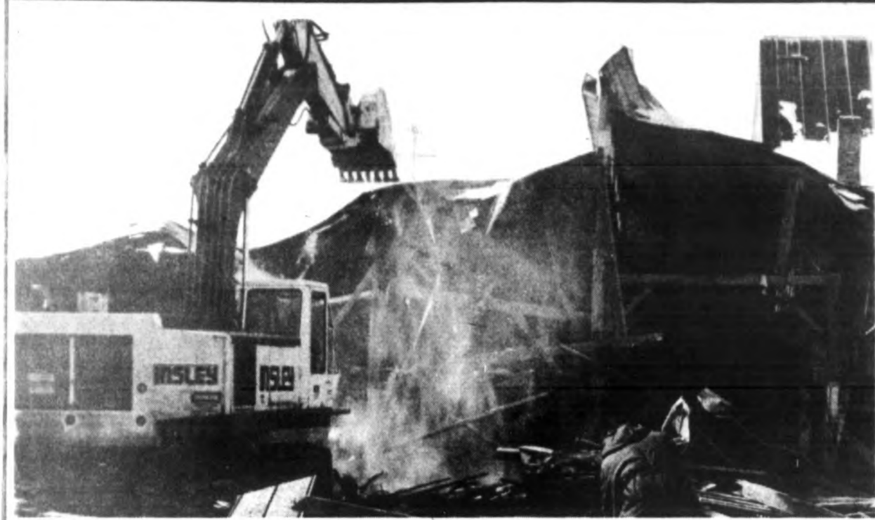
DEMOLITION — A crew from Searles Construction Company clears the old stockyards from its site along the railroad tracks. The property will be used by Central Michigan Lumber to store lumber.
