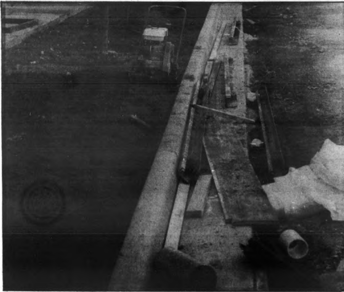
ST. JOHNS DOWNTOWN PROJECT IS MOVING RIGHT ALONG—One block at a time, construction crews tear up one sidewalk and then lay forms and pour cement for the new sidewalks. Photo by Harold Schmalz, CCN.
