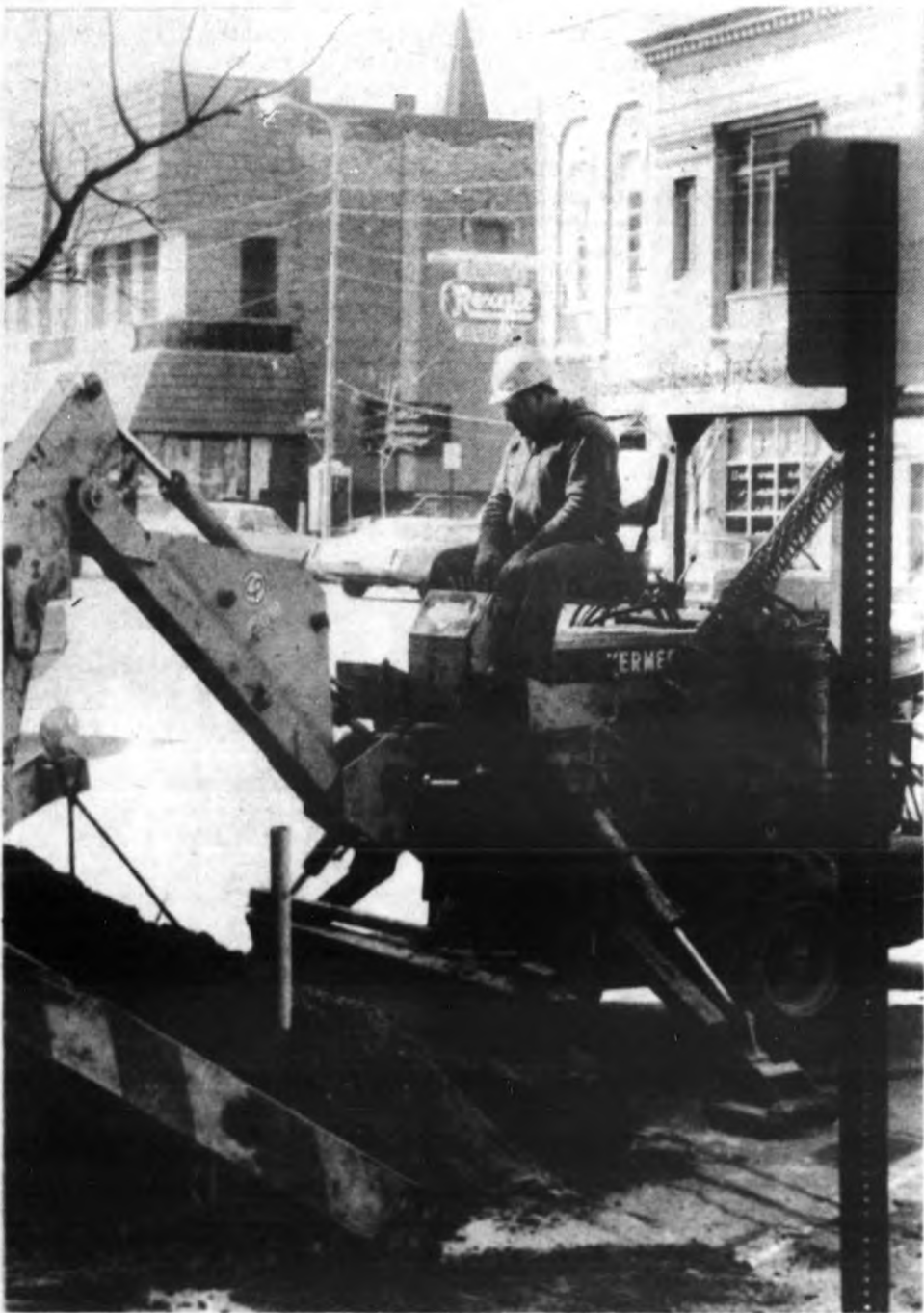
A FAMILIAR SIGHT ON MAIN STREET-Fred Smitgen replaces a two inch gas main. Photo special to the CCN by Jack Minsky.
