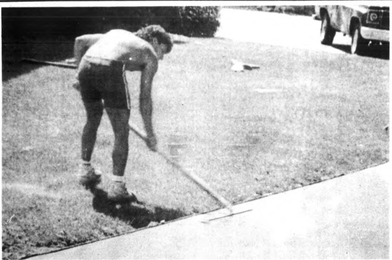
ROSS POPE spends a hot day spreading new cement in front of the First United Methodist Church on State Street in downtown St. Johns. Pope is working for the Russell Pope Construction Co. which is owned by his father. The crew has been doing some minor maintenance outside the church. Photo by Dave Holzman.
