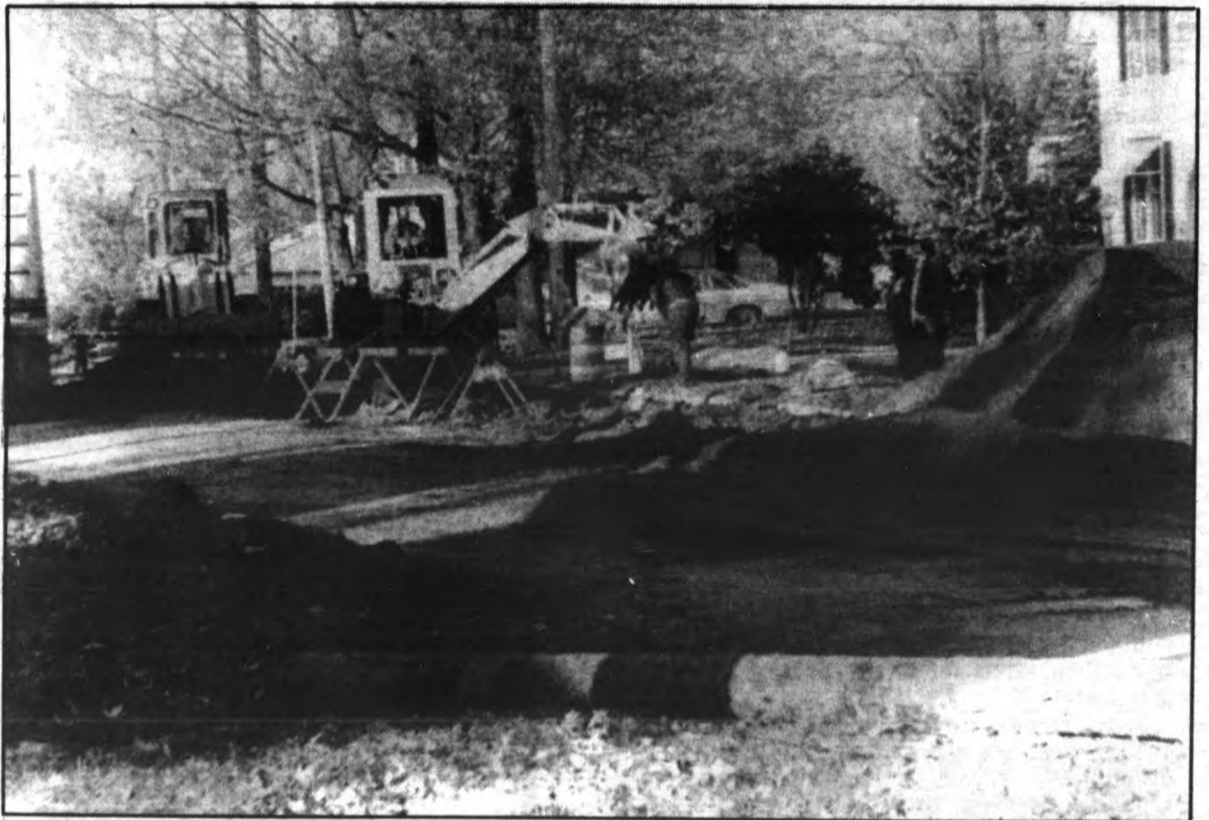
WATER MAIN INSTALLED For St. Johns residents wondering, the city crews working on Garfield Street last week were replacing a water main. Materials for the project are estimated to cost $4500. The project should be completed sometime this week.
