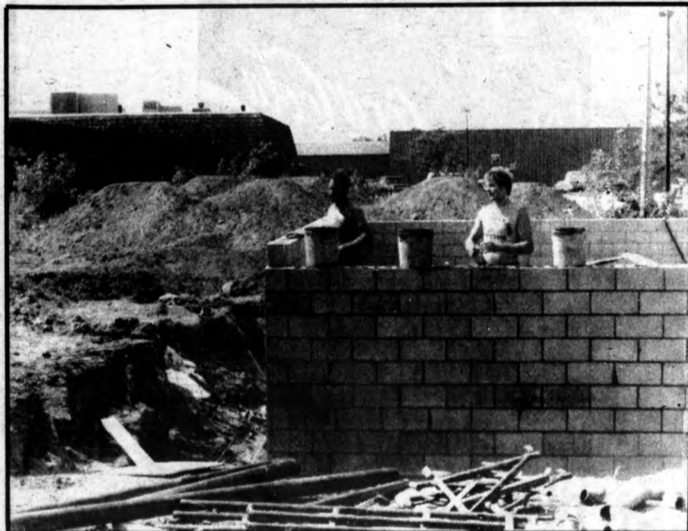
WORKERS BEGAN LAYING THE FOUNDATION for the new Wendy's Restaurant in St. Johns this week. The date of the completion is tentatively set for the end of July.
