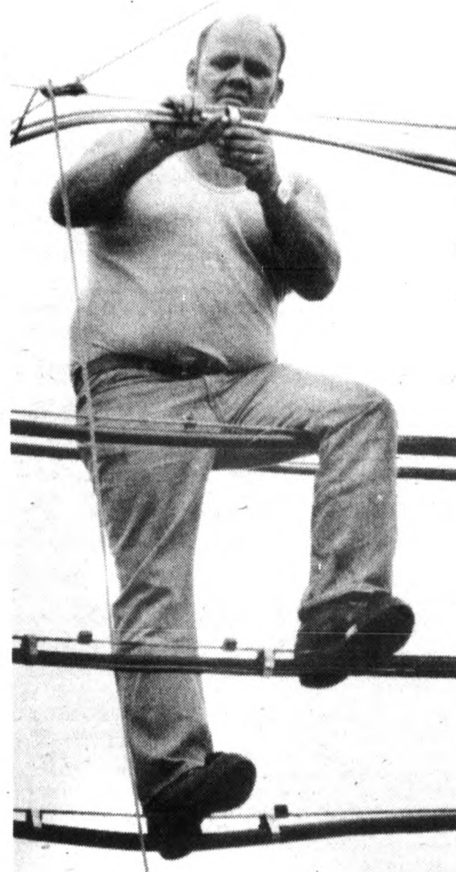
Here comes cable! Workman Jim Weishuhn attaches cable wires to existing utility poles at the corner of Turner and Heribson Roads. If work proceeds as expected, city residents will be hooked up by the end of summer. (Photo by David Olds)
