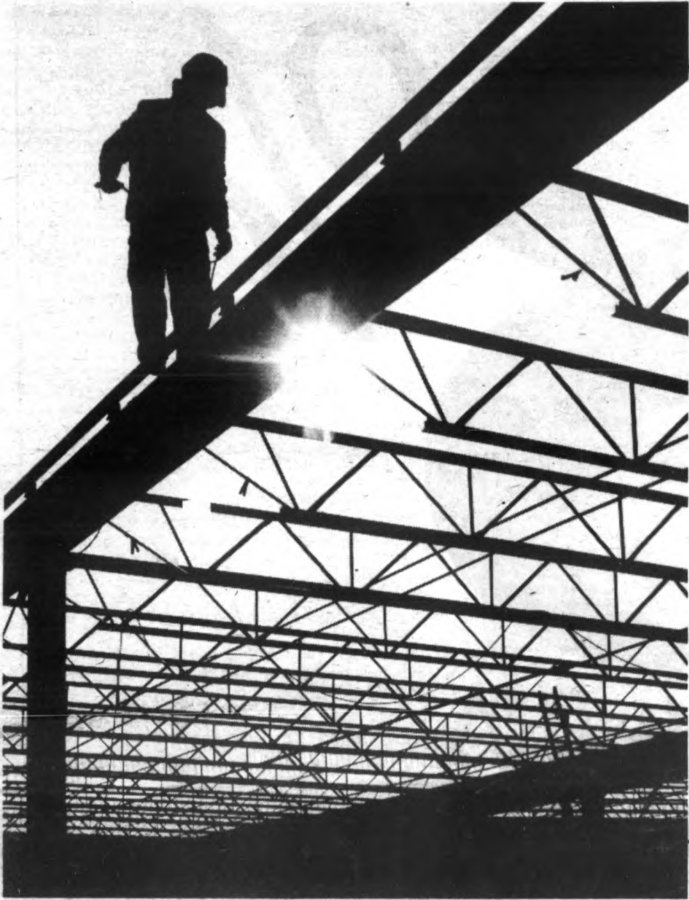
A welder, braving cold and windy weather, works his way down an I-beam at the construction site for the new mall in St. Johns.
