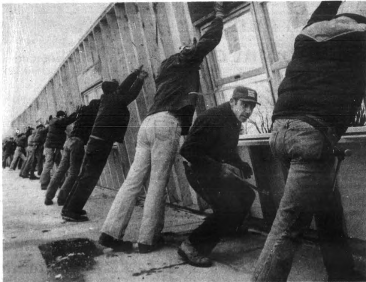
Arnold Busenitz checked the progress of more than 40 Victor Township volunteers as they raised the first wall of their new township hall last Saturday morning. The hall is being built mainly with volunteer
