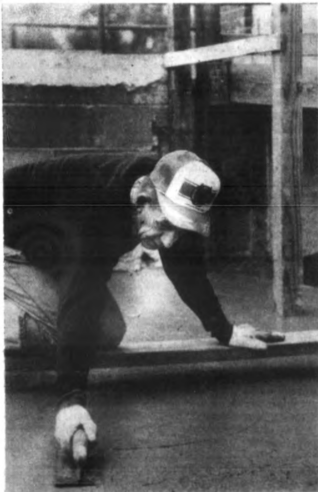
Clinton Wright and Merle Trowbridge look on as Barry (right) and Al Hartman (left) put the finishing touches on some fresh concrete at Gunnisonville United Methodist Church. They are among several volunteers who have been working for the past five weeks to install a new handicapper ramp, railings and new steps. While the work was in progress, church leaders decided to also have some improvements done to the church steeple. (Photo by David Olds)
