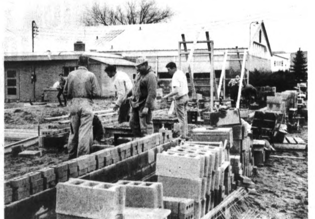
In April, 1967 the walls were going up at Eureka in one of four phases of construction on rural elementary schools in the St. Johns system. Eureka's was a 7-room addition. Foundations were already in at the East Essex addition site. Meanwhile bids were soon to be opened for construction of a new high school near the city park.
