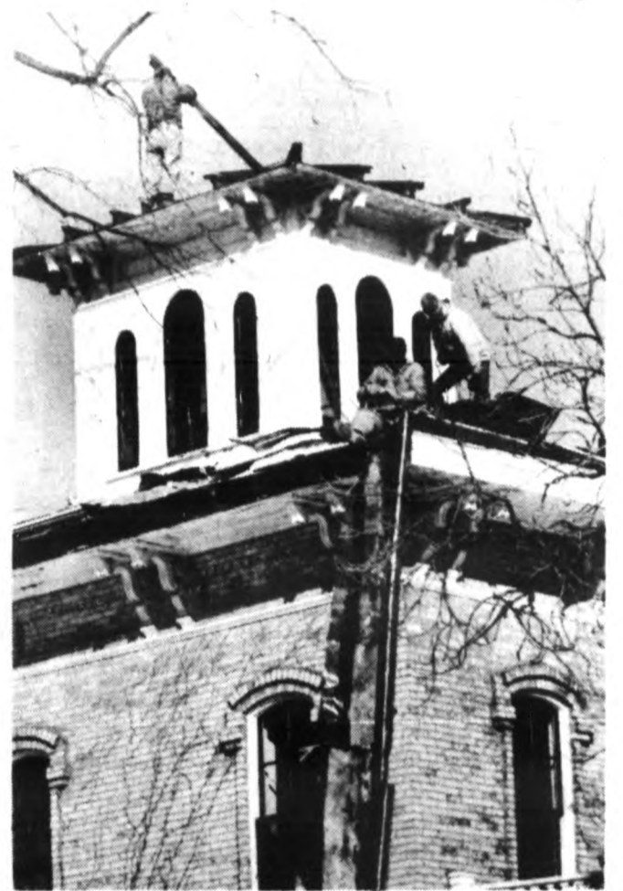
Demolition workers began razing the old Wilson home at the corner of Cass and Maple in St. Johns in March, 1967. The first step, of course, was to tear down the cupola on the roof.
