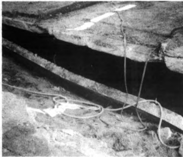
This 10 year old concrete manure structure failed while being emptied in the spring. Failure was caused by installing minimal amounts of steel rebar in the walls, coupled with excessive pressures from waterlogged backfill.
