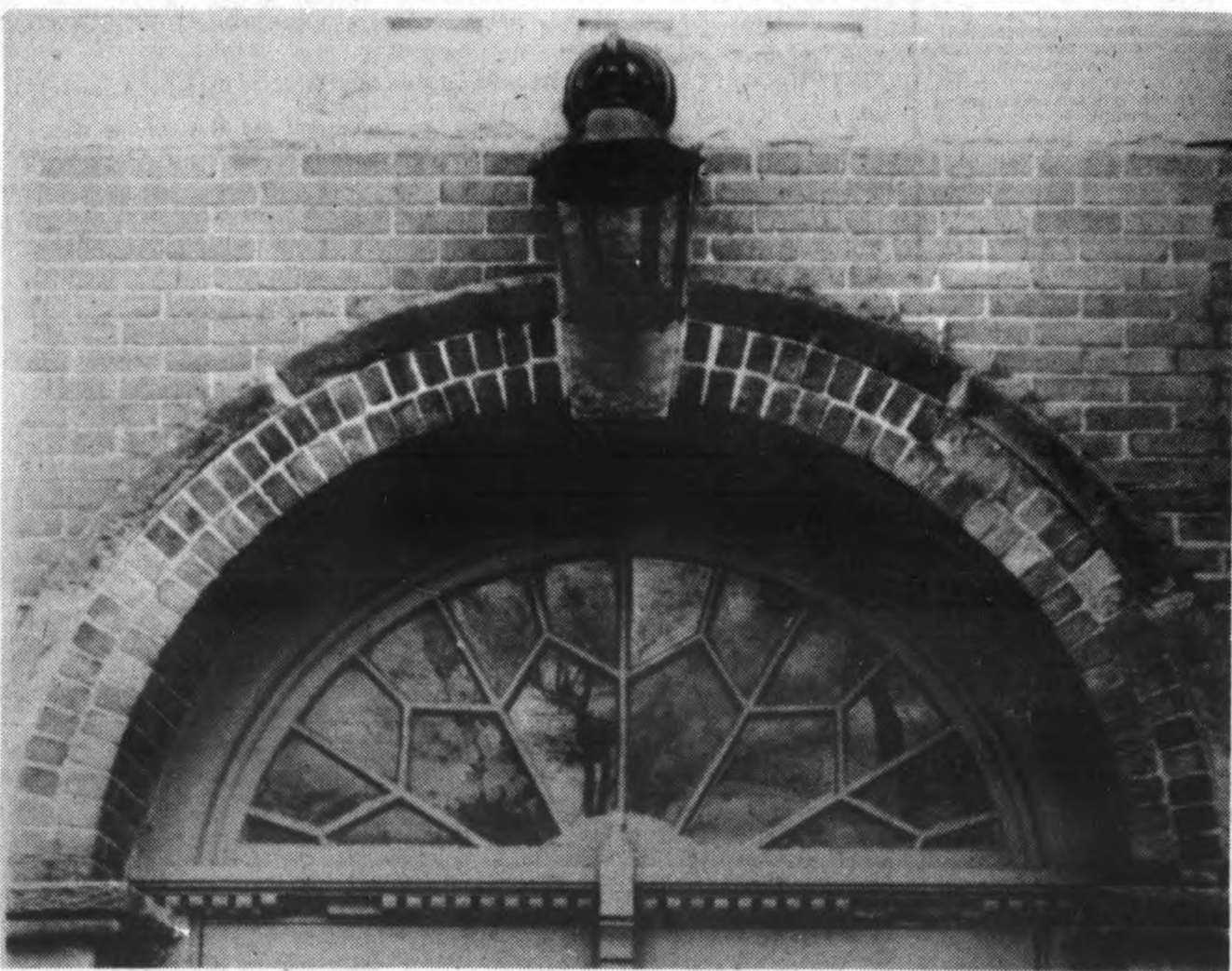
This light fixture over the fanlight window above the west main entrance is not original to the building but was added sometime after the
