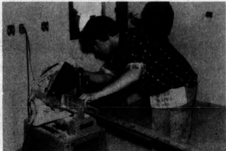
Student is Jack Smith cutting base for family room using a power mitre. This is just one of the many skills Jack has learned in his two years in Building Trades.
